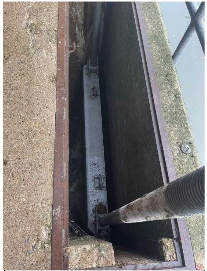
Photo 0060811042466 - Slide gate bay number 2
