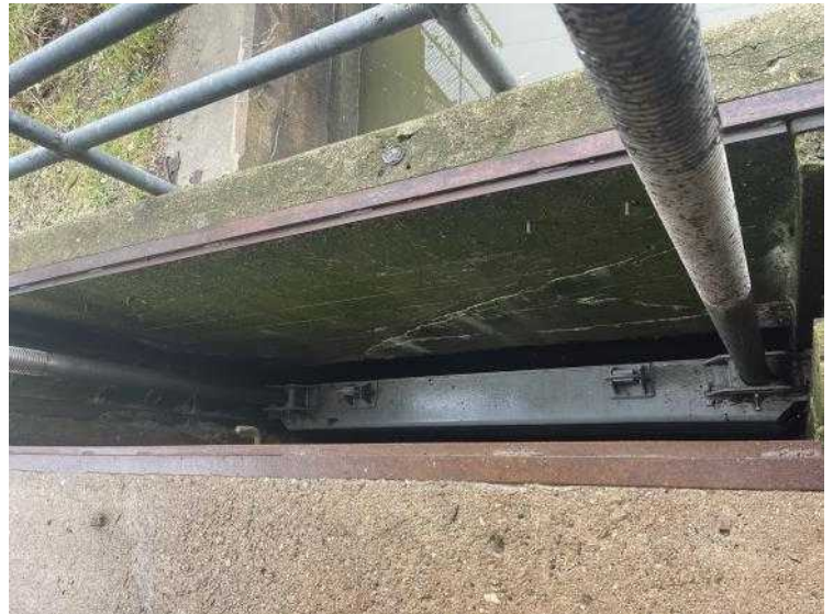
Photo 0060811042462 - Slide gate bay number 6
