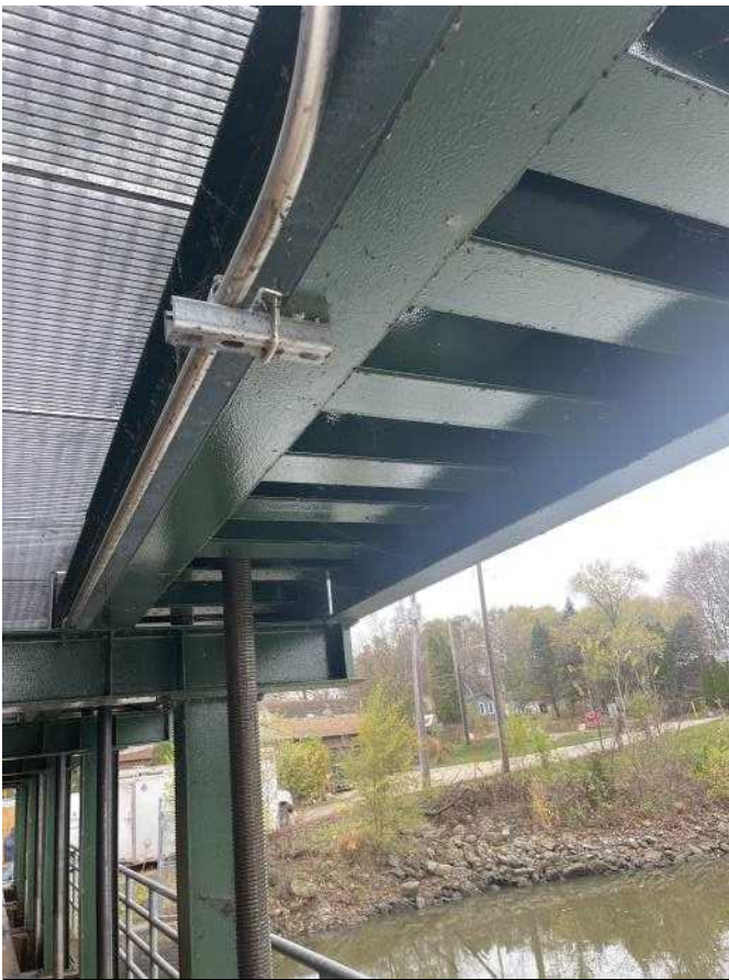
Photo 0060811042469 - Slide gate platform beams
