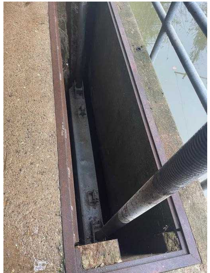
Photo 0060811042464 - Slide gate bay number 4
