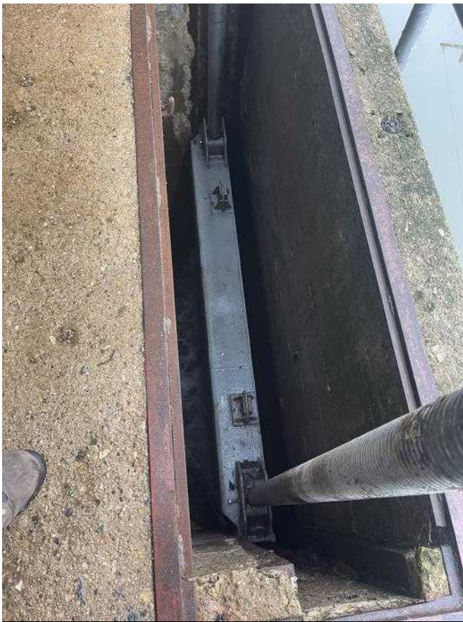
Photo 0060811042465 - Slide gate bay number 3
