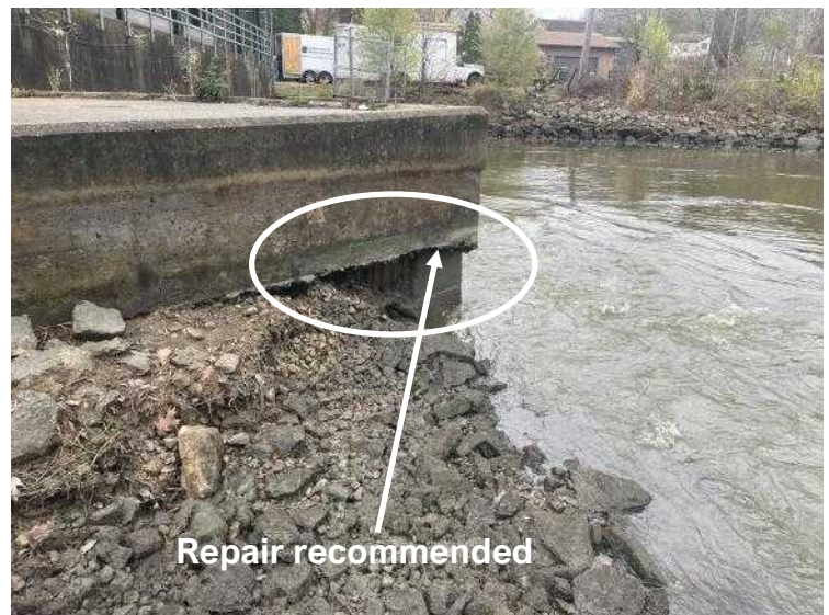
Photo 0060811042432 - Scour at primary slide gate abutment
