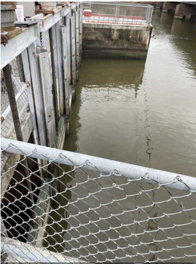
Photo 0060811042406 - Auxiliary slide gates (up river)
