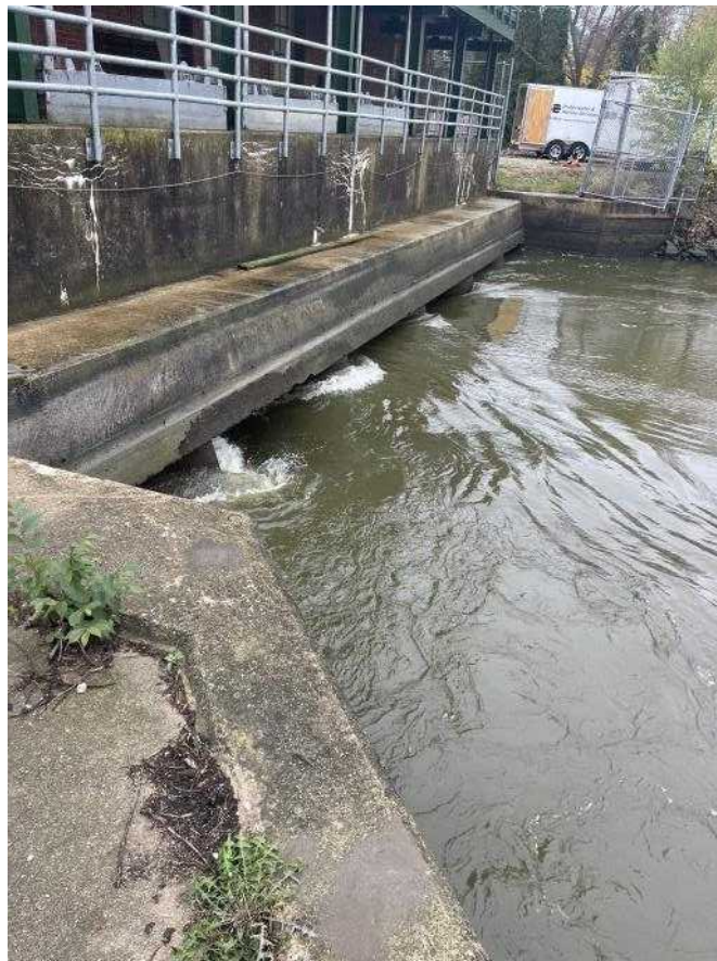
Photo 0060811042435 - Primary building slide gate intake
