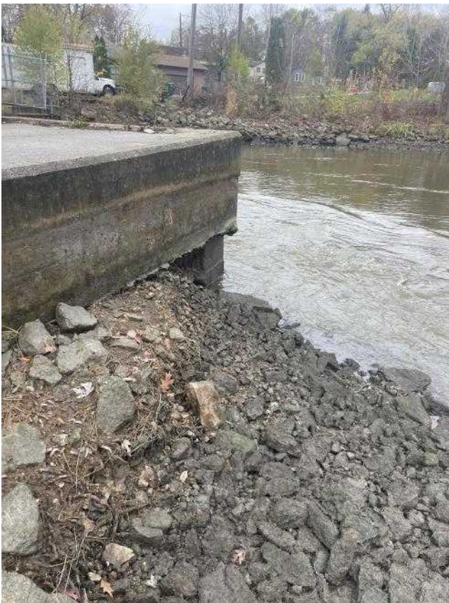
Photo 0060811042431 - Scour at primary slide gate
