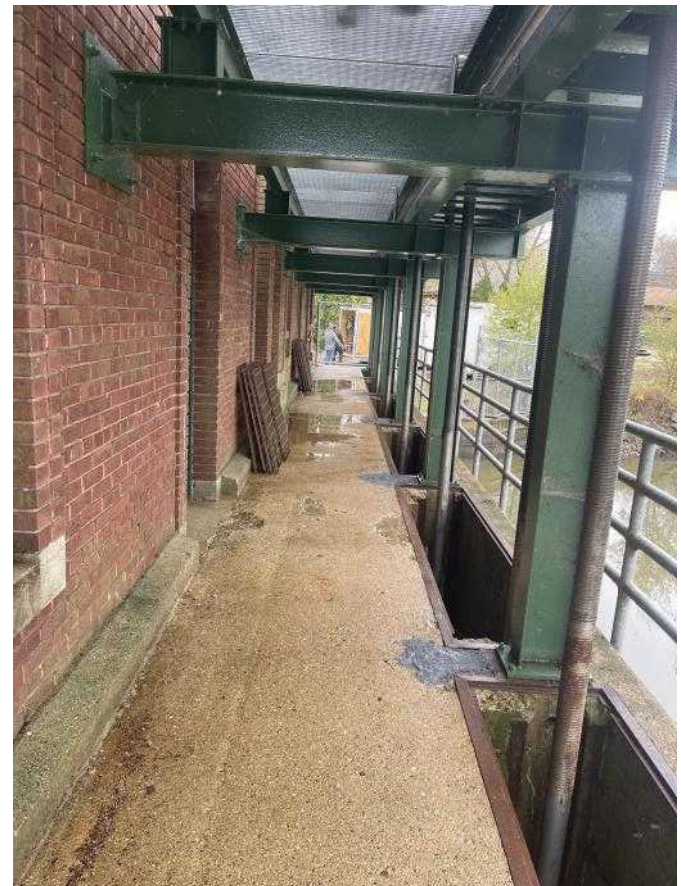
Photo 0060811042468 - Slide gate platform (looking west)
