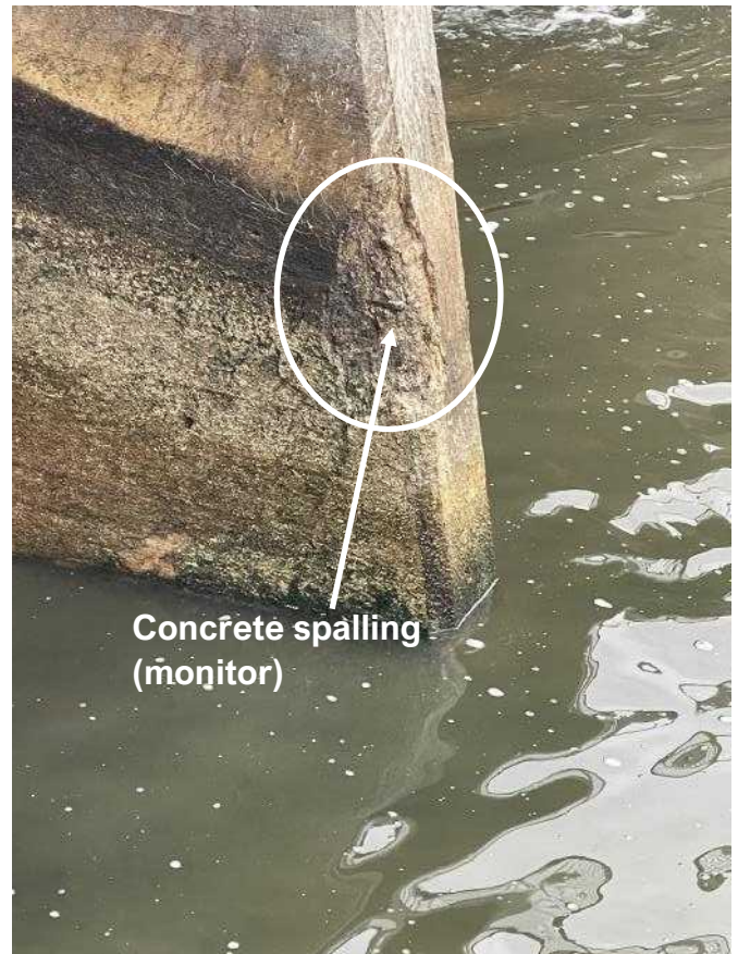
Photo 0060811042417 - Monitor concrete spalling at third
