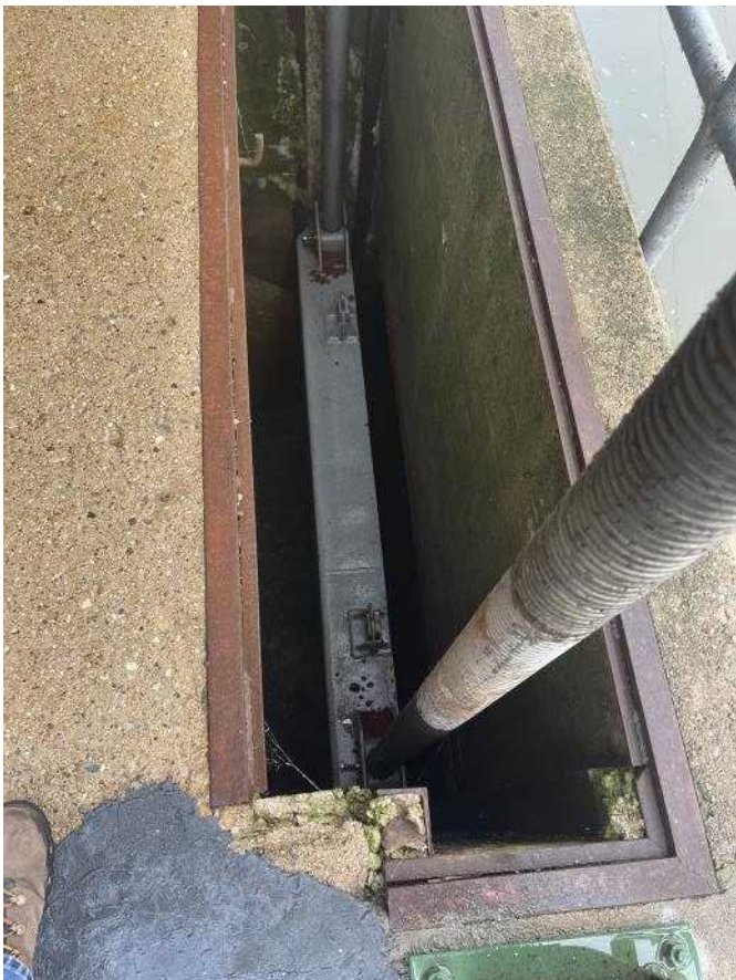
Photo 0060811042467 - Slide gate bay number 1
