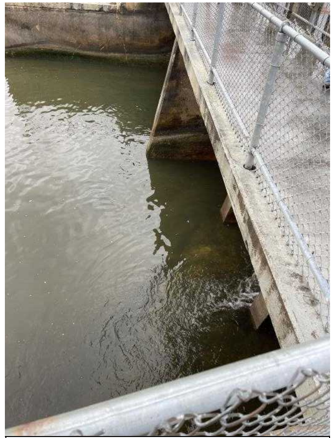
Photo 0060811042407 - Auxiliary slide gates (down river)
