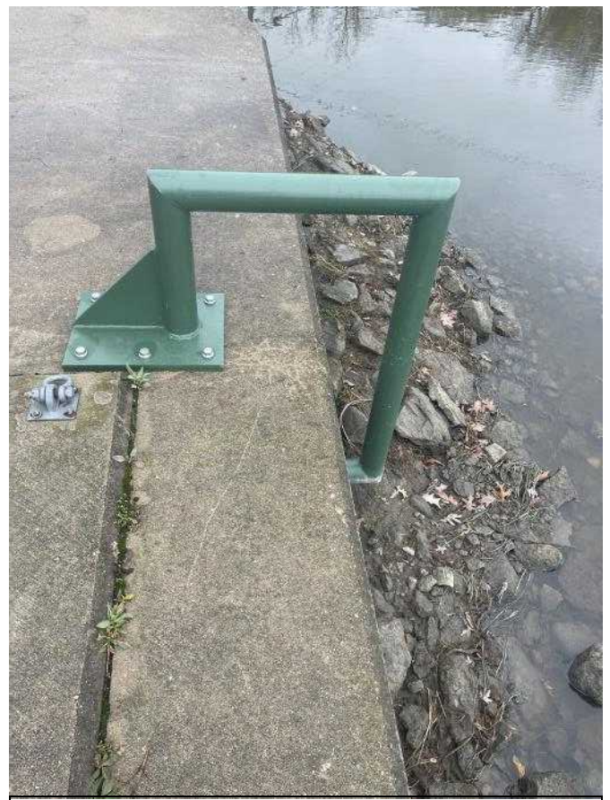
Photo 0060811042454 - Down river debris boom anchor
