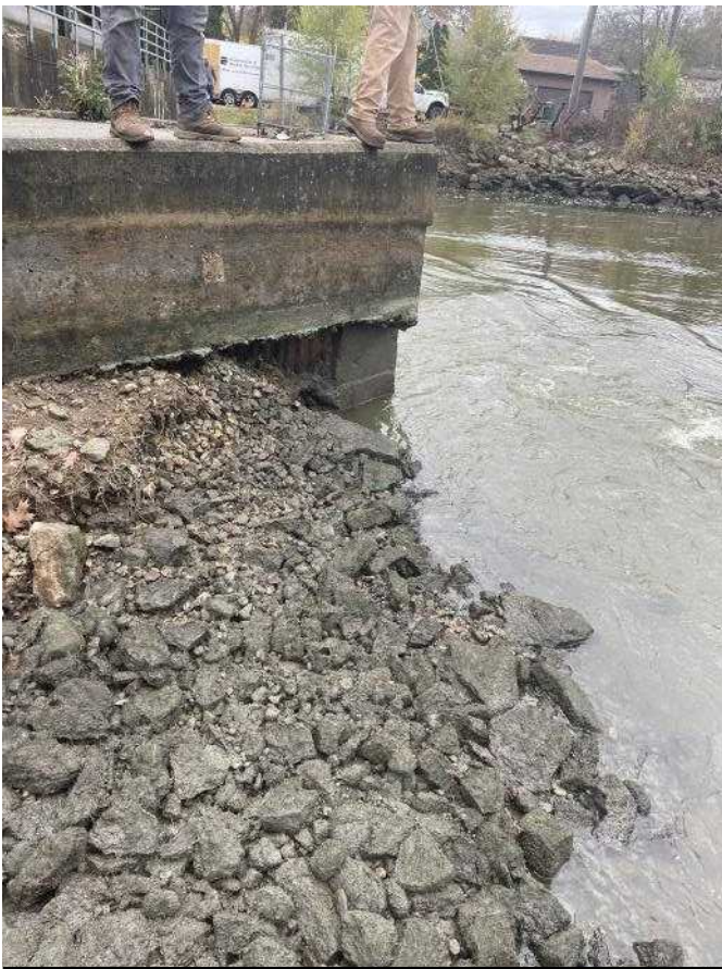
Photo 0060811042433 - Abutment scour at draw down
