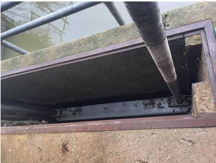
Photo 0060811042463 - Slide gate bay number 5
