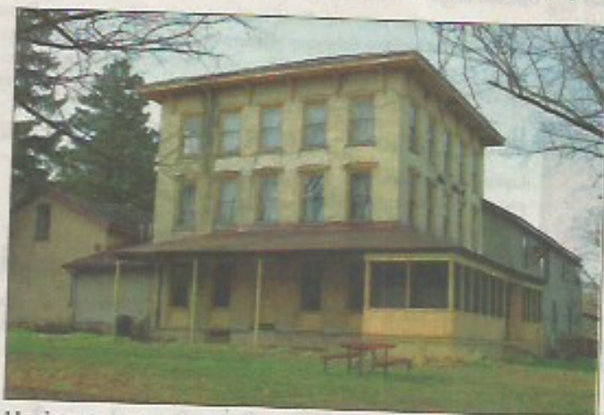
Having recently gone out of business, The Lake House Inn sits empty this holiday season. The historic building awaits its next chapter and faces much-needed renovations and repairs.
