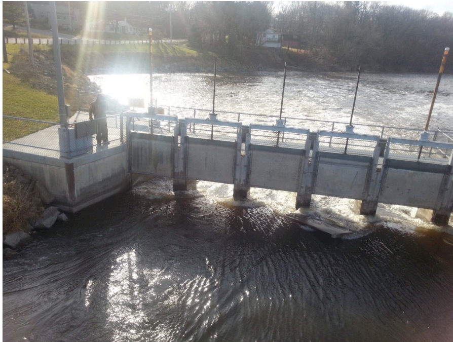
Photo 0060812051302 – Three missing stem covers
