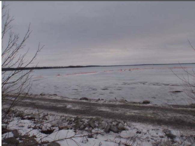
At the staging area, looking south onto the eastern side of the dredge area.
