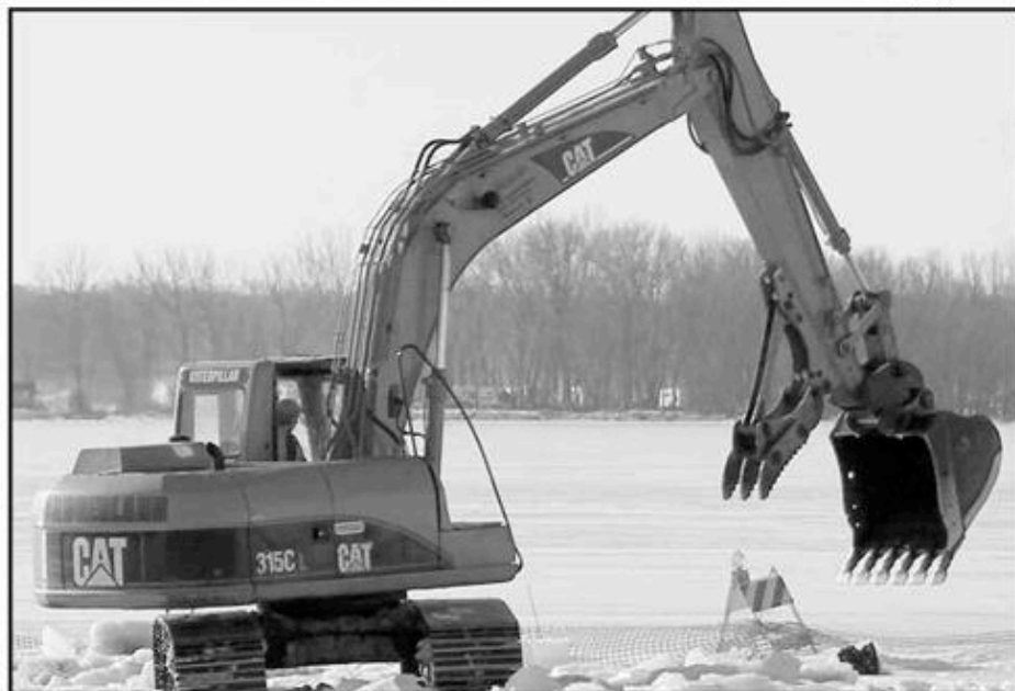
A year-long experimental dredging project by the Rock-Koshkonong Lake District is complete. In this photo an excavator pulls up slabs of ice last February.
