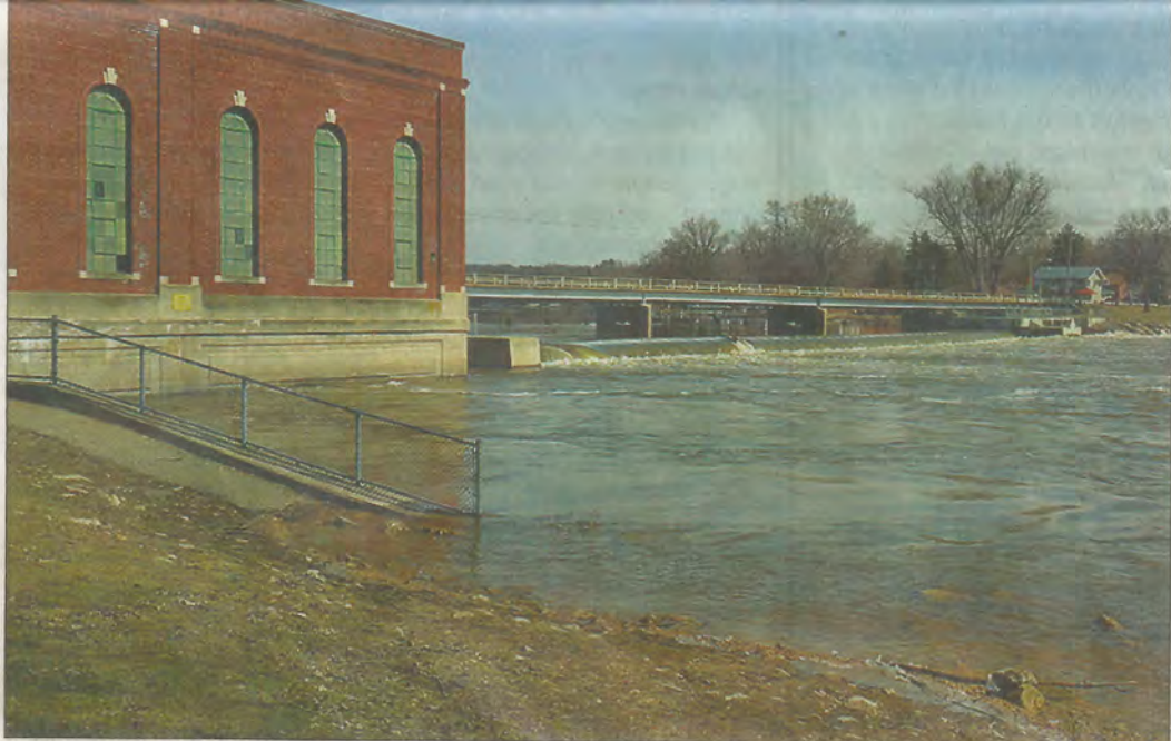
The Rock River bridge in Indianford has a badly deteriorated deck, which will be replaced next year.
