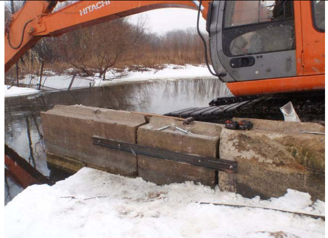
At the carp gate looking south onto the construction. The strapping has been anchored to the concrete blocks.
