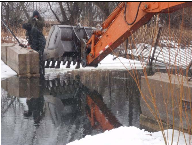
At the carp gate looking east onto the installation of the anchorage poles.
