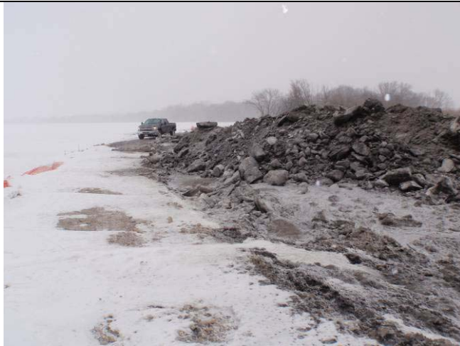
At the south end of the berm looking north onto the dredge placement area.
