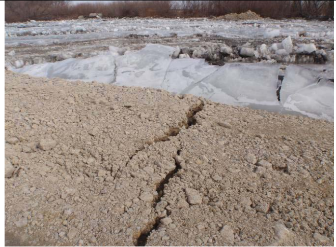
At the south end the berm looking at a crack caused by the ice heaves.
