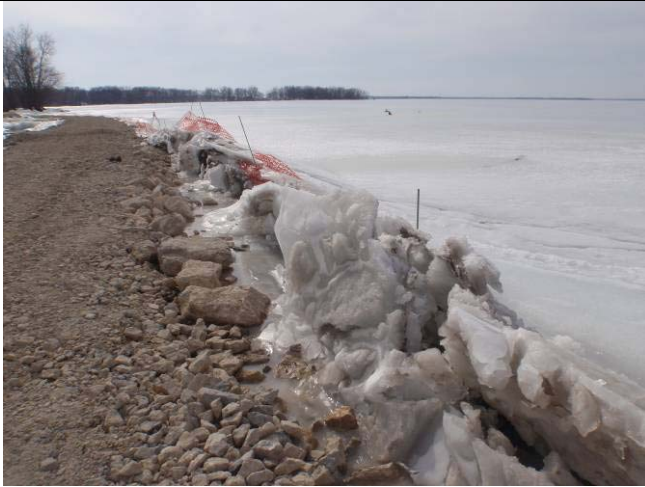
At the north end the berm looking SW at the ice heaves.
